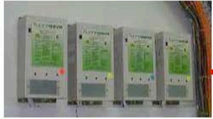
Power Saving Device (PSD)
