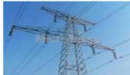
Transmission & distribution loss
